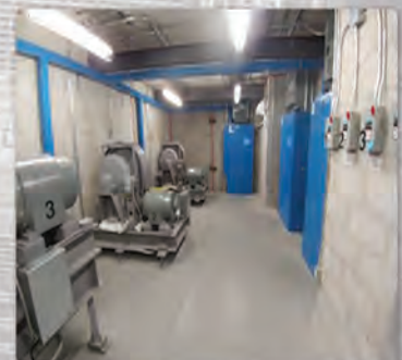
Machine Room Is Required
